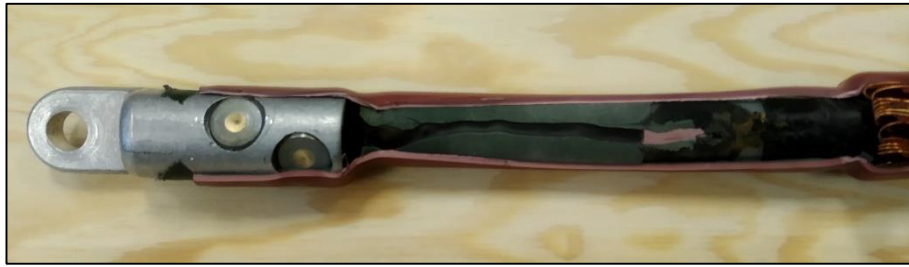
Fig. 72 Breakdown path from wire screen to cable lug through stress-grading material layer – the typical situation for samples T4-T9 (Reproduced from [A1])
